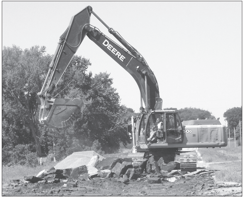
Work continues on large culvert replacements at three locations on Minnesota Highway 30 between Blooming Prairie and Ellendale. The detour is expected to be in place for about another week.
